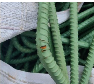
Don't field bend epoxy rebar
